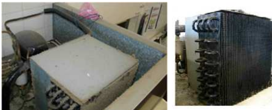
Figure 3-2: Top mounted condenser on plug-in service cabinet prior/after cleaning
